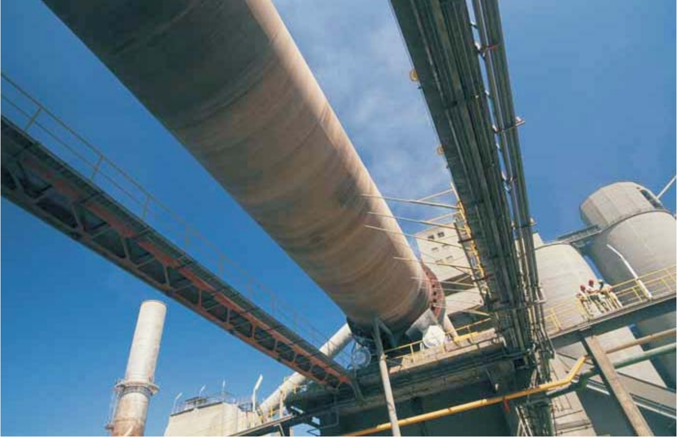
Rotary Kiln with DC-Motors
