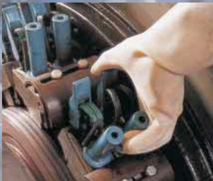
Individual plug-in brush holders are grasped by the insulated handle lever. For safety reasons, safety gloves should additionally be used during this procedure.
